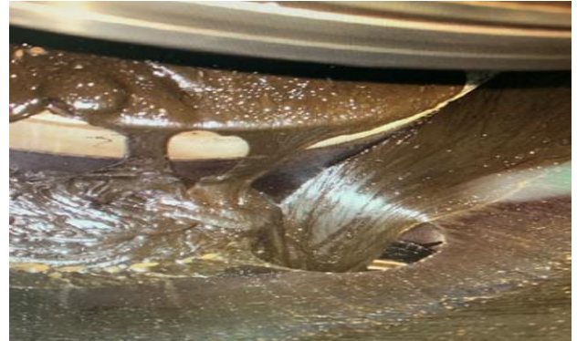
Waxy fuel blocking centrifugal purifier drains
